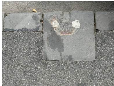
Figure 23. (right) Large kerb block with remnant marks where a verandah post was fixed (City of Ballarat, January 2023).
