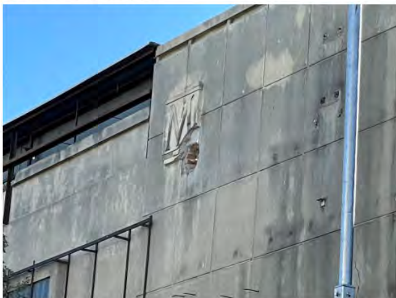
Detail of the c.1952 façade showing the original 'M' logo, incised grid pattern, parapet capping shadowline detail, and evidence of the original flagpole fastenings to the right.
