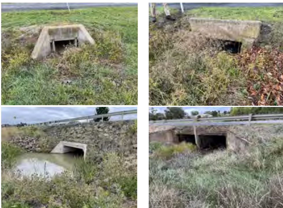
Figure 12. Photo of a typical road crossing of the waterway in the North-west growth area
