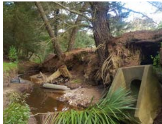
A heavily degraded waterway in Ballarat’s East
