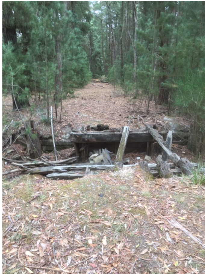
The old rail bridge over the creek. The plan is to place a modern bridge over the old works without damaging the heritage values and remnants of the old bridge. Looking north.
