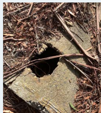
4. Damaged septic tank. (Odours, water ingress leads to failure)
