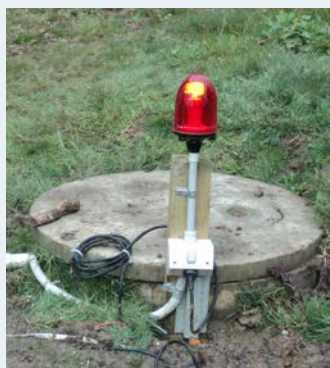
2. Flashing alarm triggered indicating pump failure.
